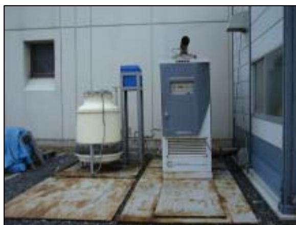
Micro gas turbine
