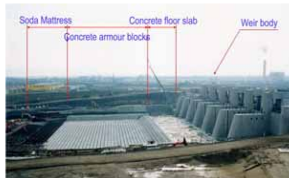
Pic. 2 Soda Mattress installed at weir (At Okouzu-Bunsui weir on Shinano River)
