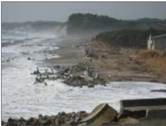
北追川沿岸護岸は津波で流失
